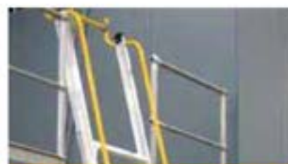
A Safety Gate is provided at the upper floor level to maintain the integrity of the perimeter railing.
